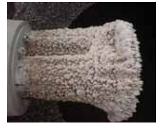
Outer unit is coated with build-up from dust.
